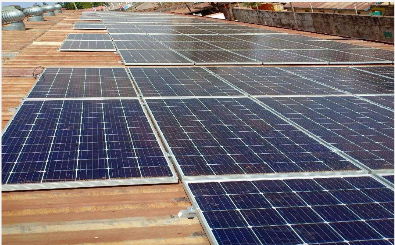
Juja, Kiambu – 36.7 kWp Roof Mount System
