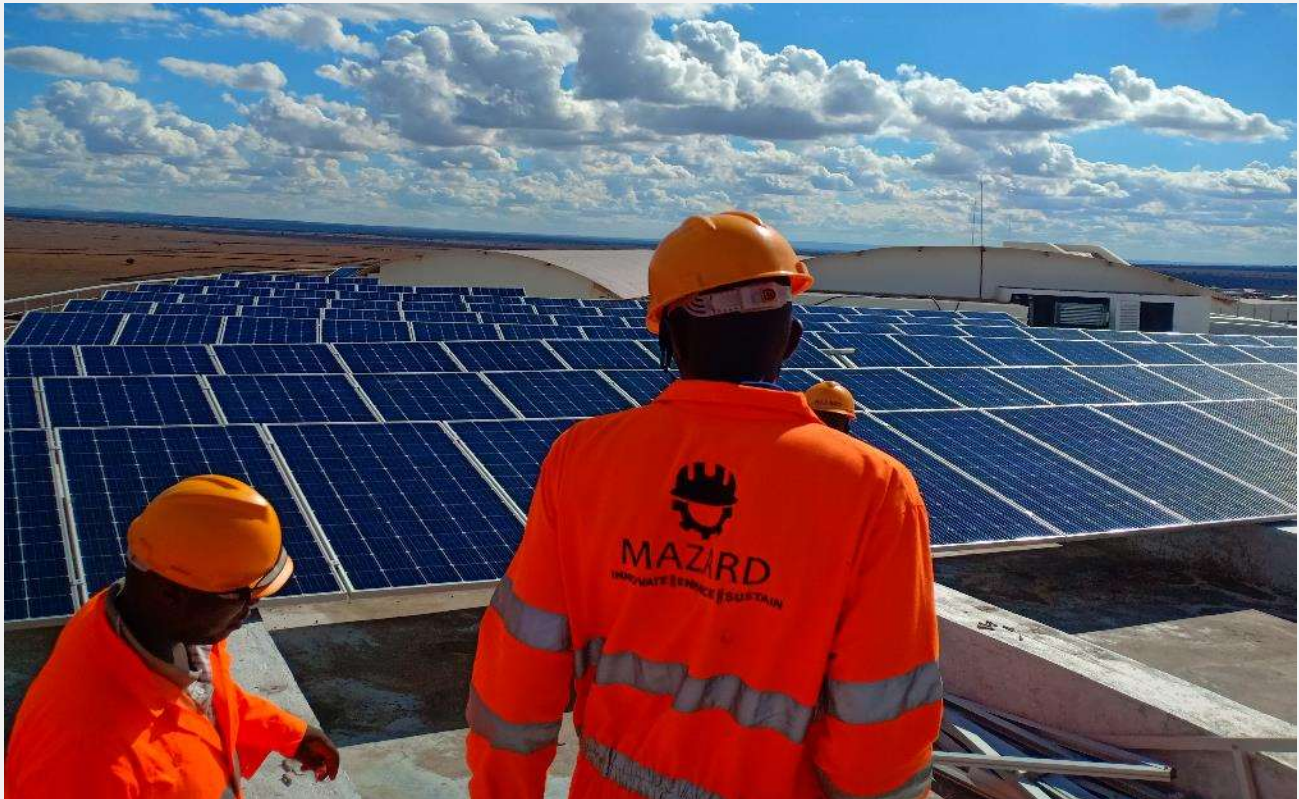
Konza City, Kajiado – 80 kWp Concrete Roof System
