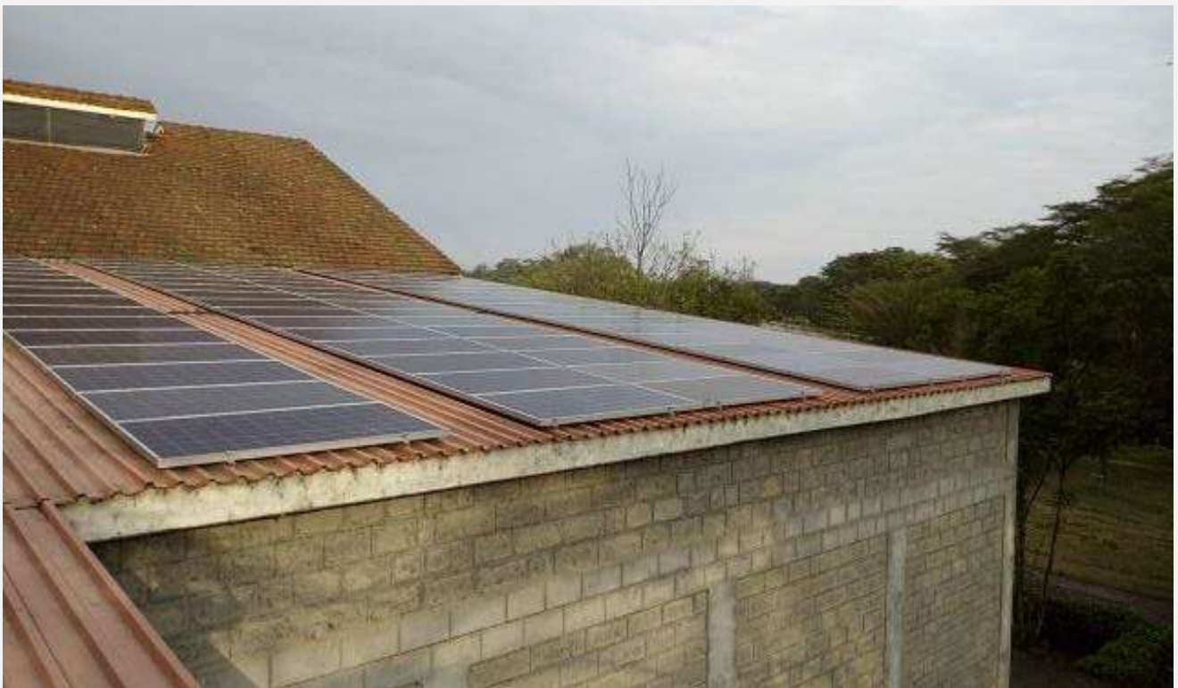
Naivasha – 186 kWp Rooftop System
