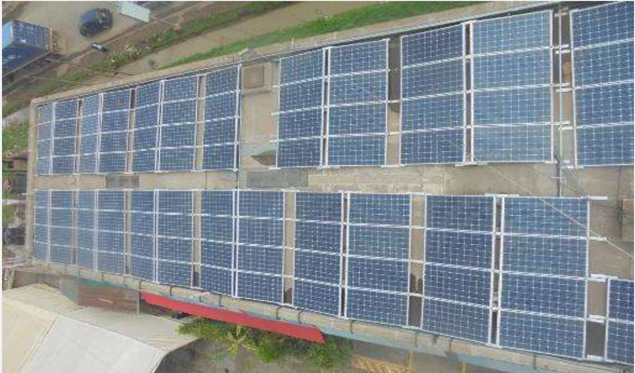
Industrial Area, Nairobi – 30 kWp Ballast Rooftop System
