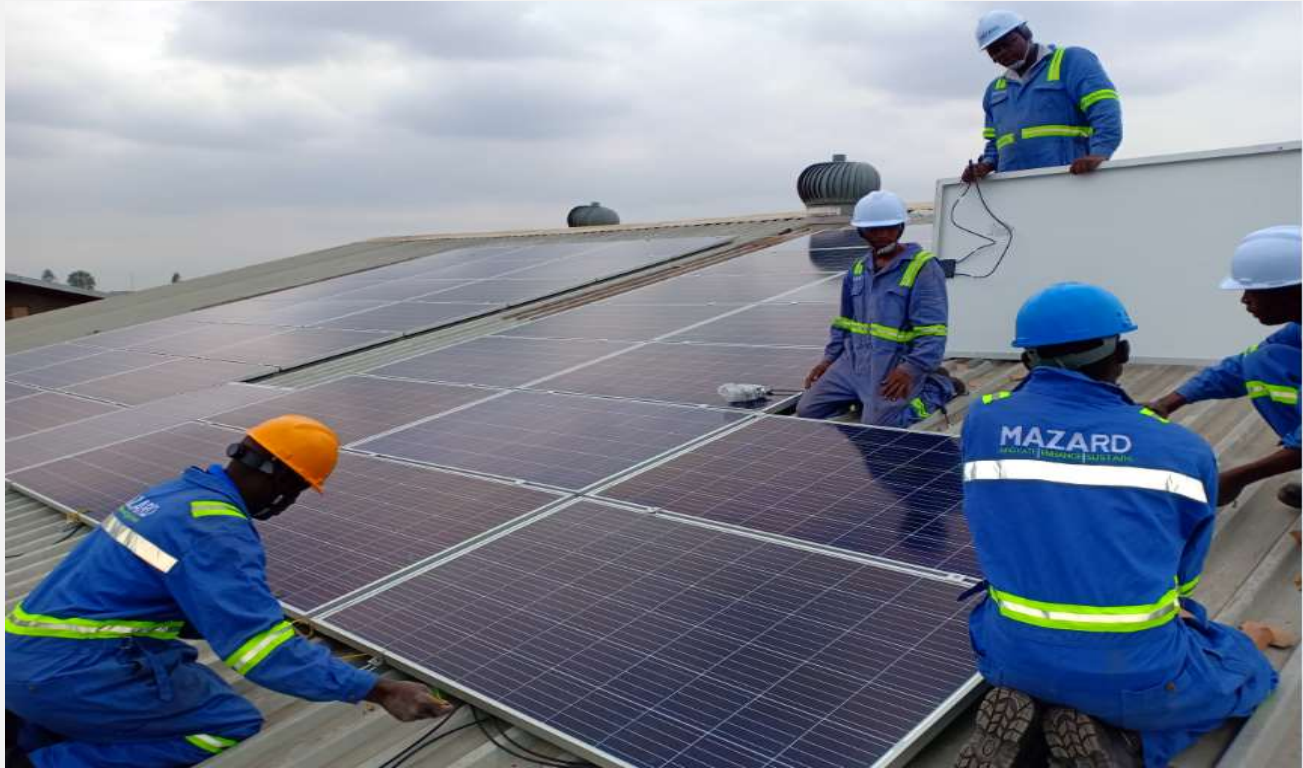
Mombasa Rd – 24 kWp Rooftop System
