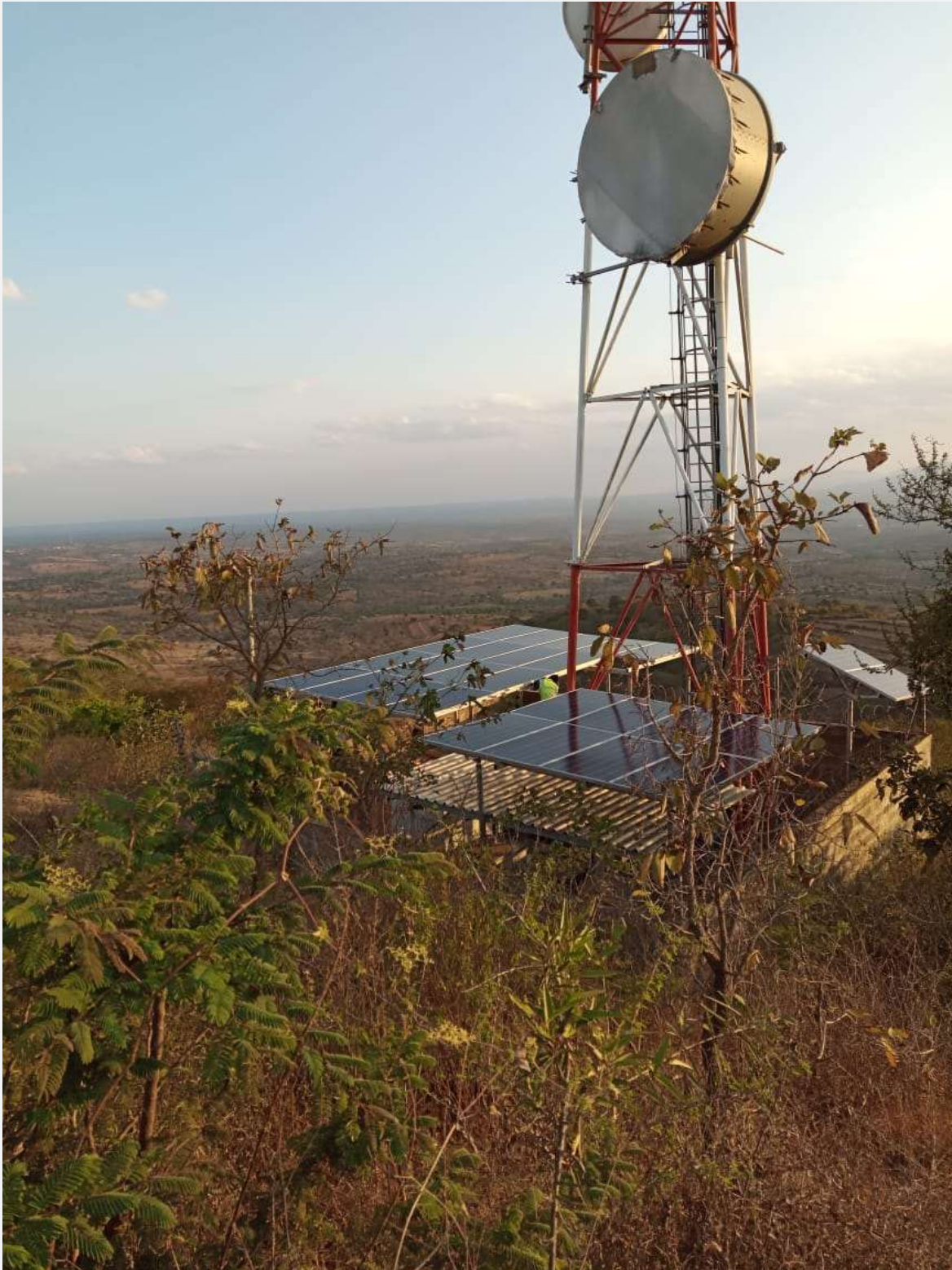
Solar Battery Diesel Hybrid – 11 Stations for Eaton Towers on behalf of Autarsys E.A
