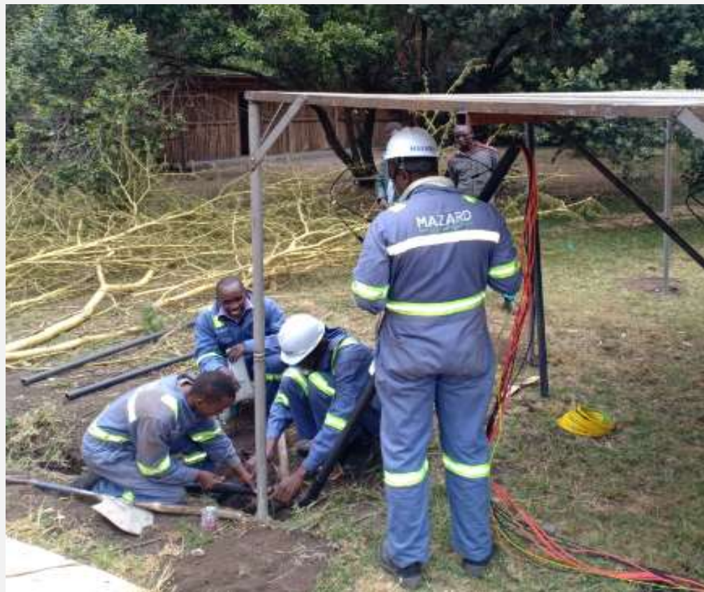
Masai Mara – 5kWp Solar Battery Diesel System
