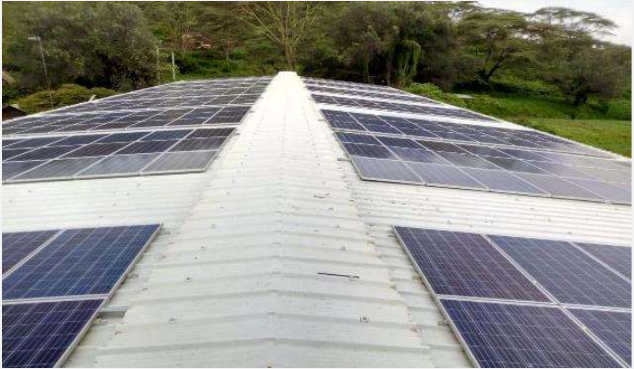
Naivasha – 186 kWp Rooftop System
